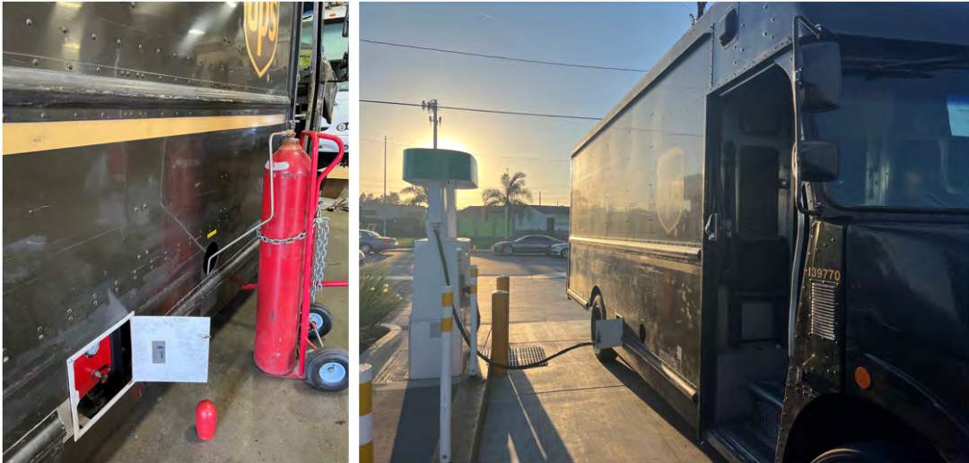
Figure 6: H2 System Commissioning, Las Vegas and Torrance
