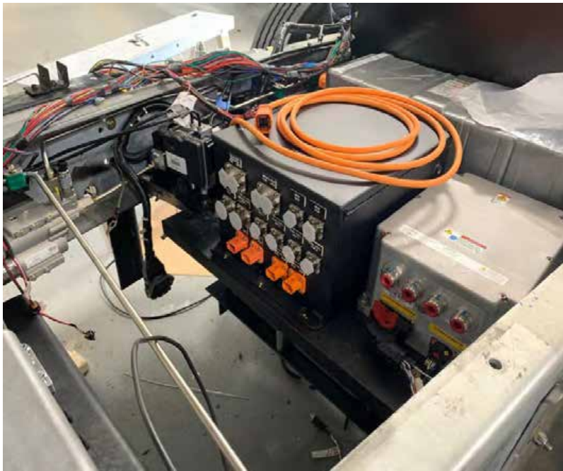
Figure 15: High Voltage Junction Box
