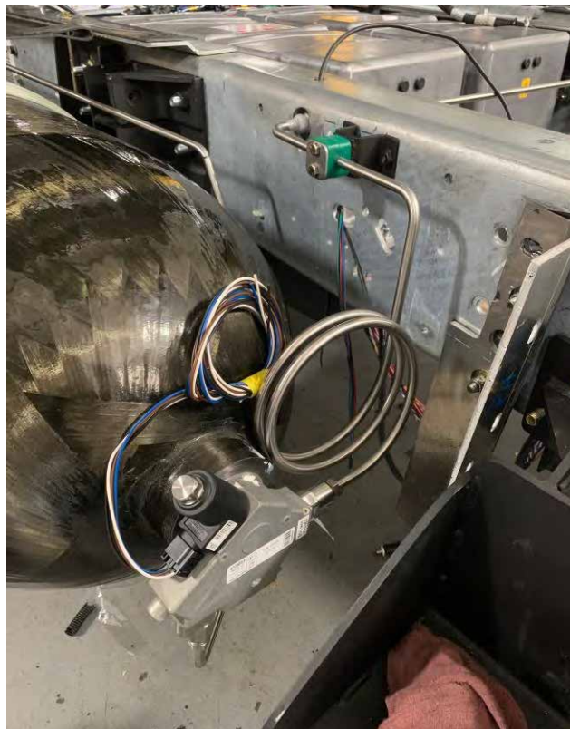
Figure 16: Hydrogen Tank Showing OMB Valve
