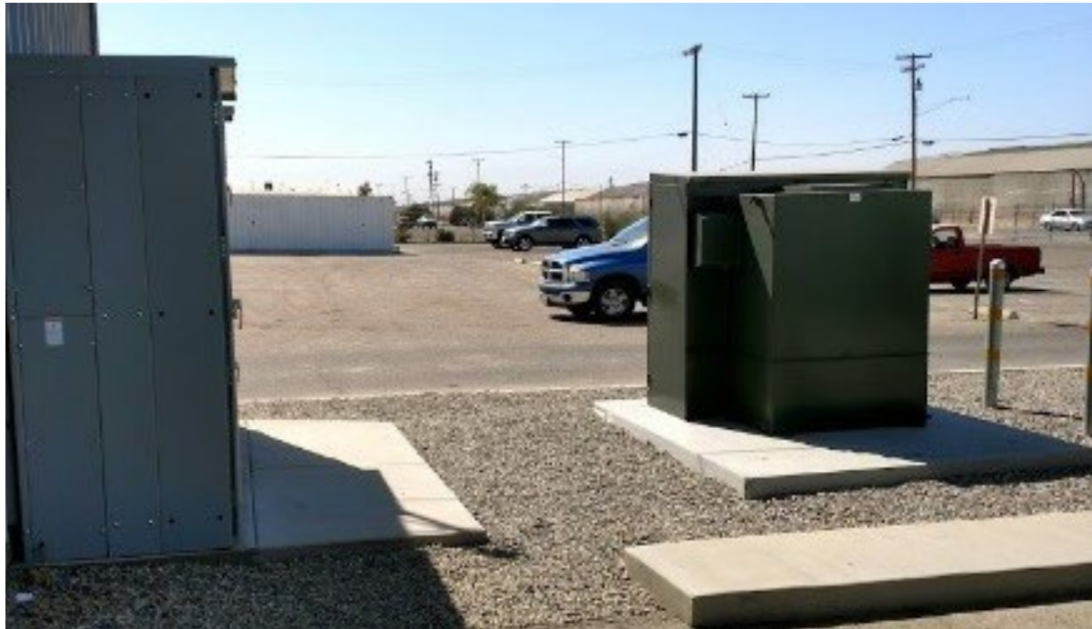
Bakersfield Pad-mounted Transformers
