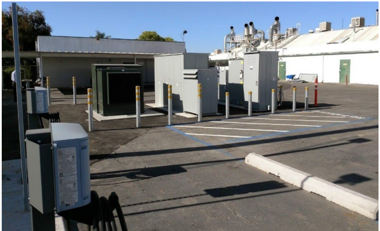
Fresno Pad-mounted Transformers
