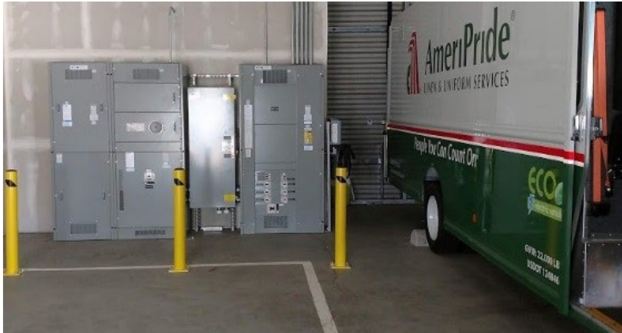
Merced Pad-mounted Transformers
