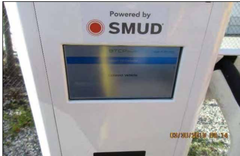
Figure 10: SMUD Charging Panel
