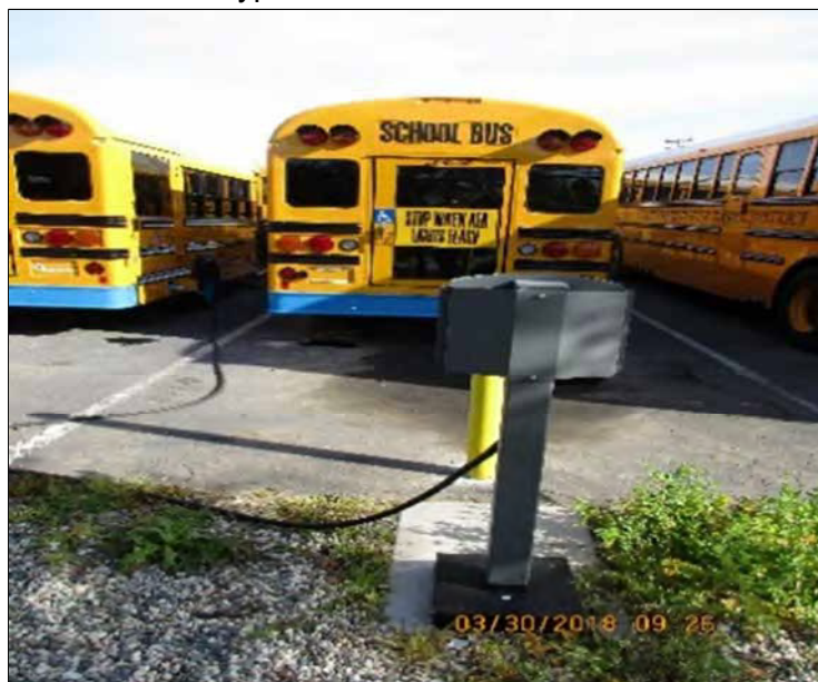
Figure 8: ClipperCreek Charging Station
