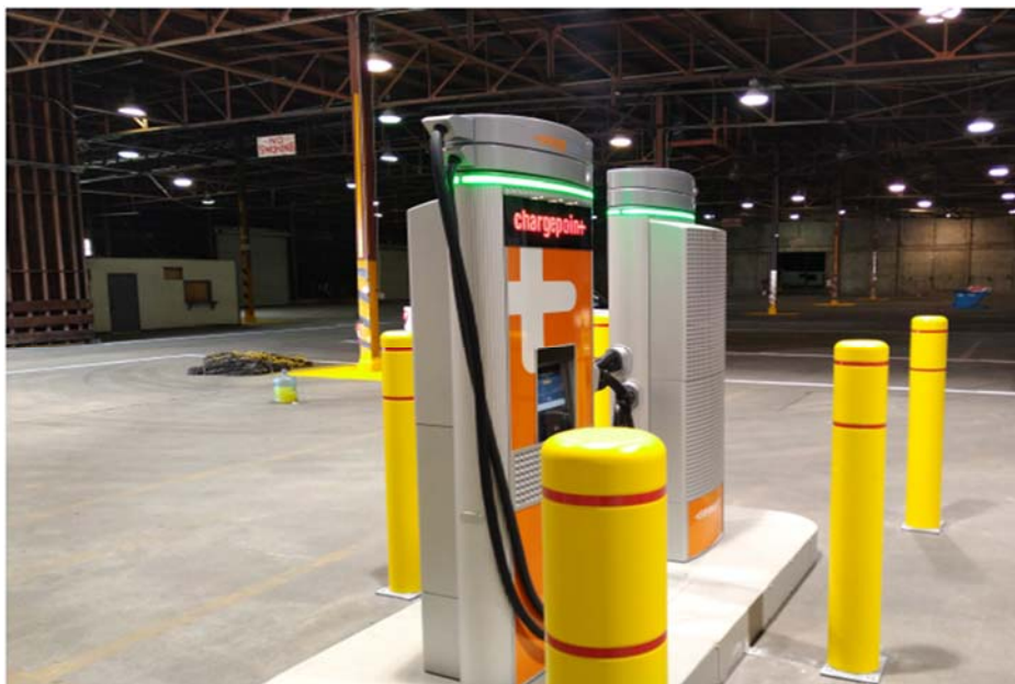
Note: Side view of the two DC fast chargers installed in warehouse 17 at the Port as part of the Project. Two yellow bollards were placed in between and one on each side of the chargers to serve as physical and visual barriers.
