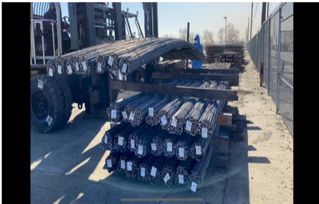
Note: Port operator discharging rebar at the Port's designated drop-off location using the DANNAR MPS with the dump bed attachment.
