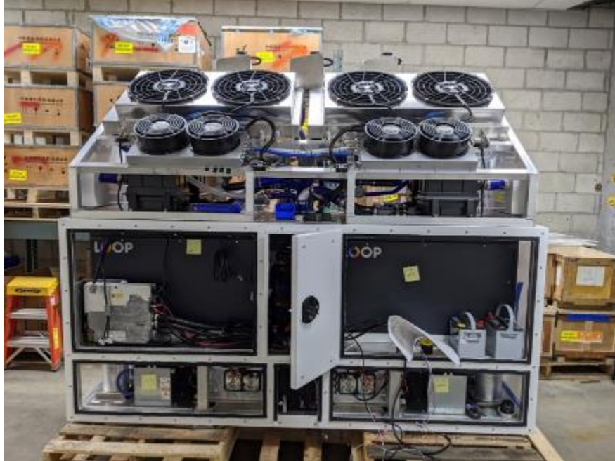
Figure 11 - Loop Fuel Cell System after commissioning
