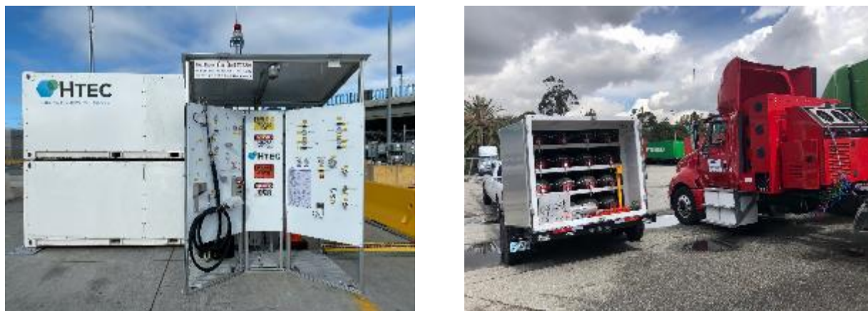
Figure 40 - Examples of Temporary and Mobile Hydrogen Fuelers
