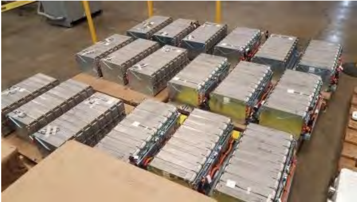
Figure 13: Assembled Battery Modules Prior to Installation into Frame Rail Cases
