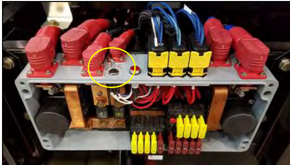
Figure 18: Inside the low voltage power distribution box. Switch circled.
