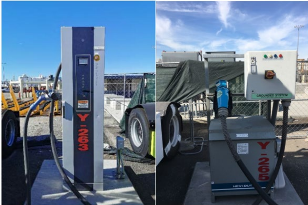
Figure 5: BYD and TransPower Chargers
