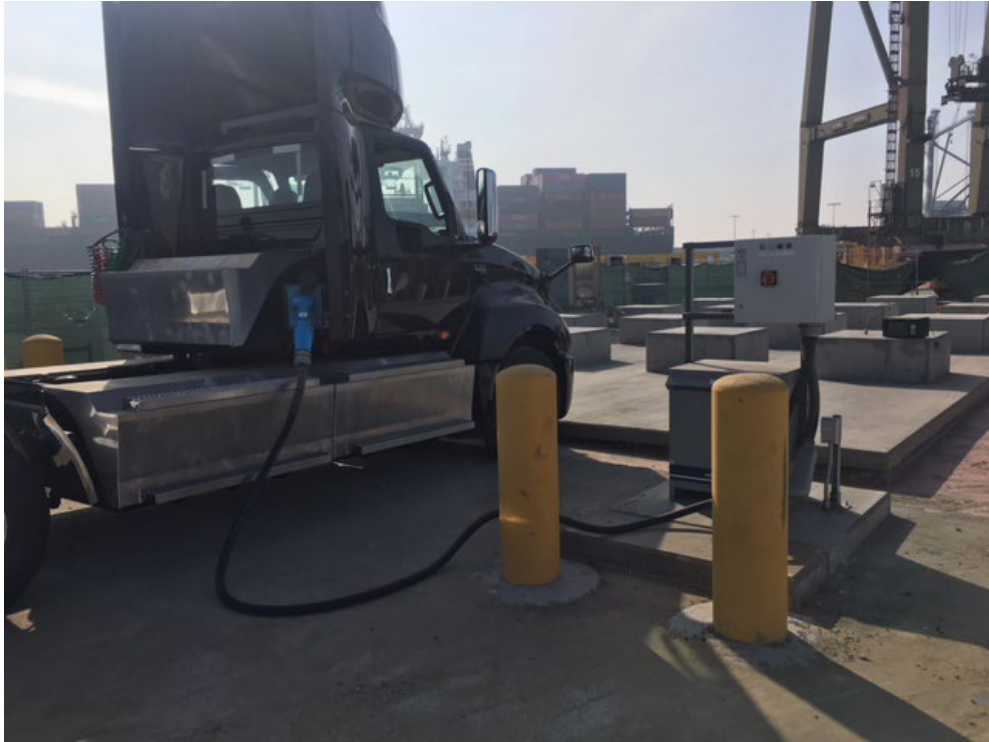
Figure 10: TransPower Repowered Battery Electric Navistar International Drayage Truck
