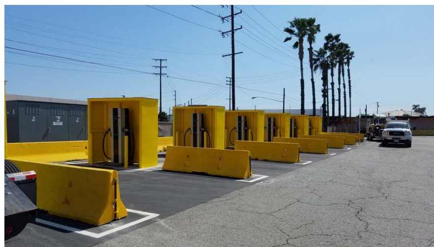
Figure 2-6: Completed EVSE Installation at BNSF-Hobart
