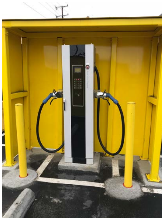
Figure 2-5: EVSE Environmental Cover Installed over BYD 200 kW EVSE at BNSF-Hobart
